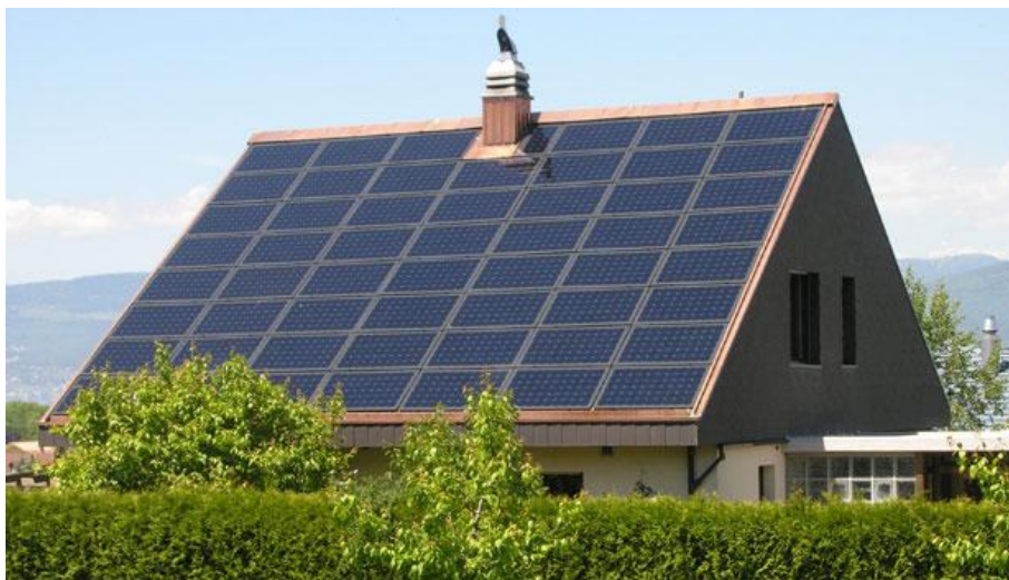
Figure 45: 'Megaslates' PV-panels on the roof of a house. From World Technology Corporation ( http://www.sunslates.net ).
