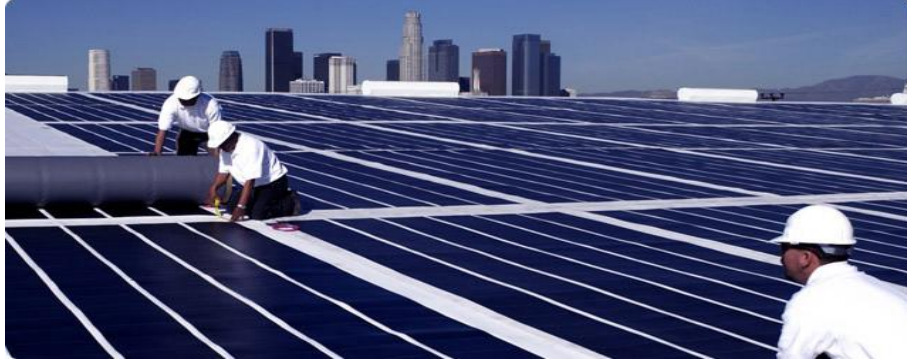
Figure 46: The Coca-Cola building in Los Angeles is equipped with 375 kW flexible thin film PV panels from UNI-SOLAR. The photo shows the panels being rolled out on the roof. Source: www.uni-solar.com .
