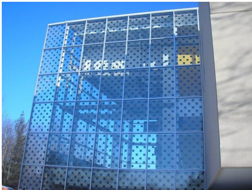
Figure 41: Solution for PV combined with daylighting, atrium in Kankakee from Atlantis Energy Systems ( http://atlantisenergy.com ).
