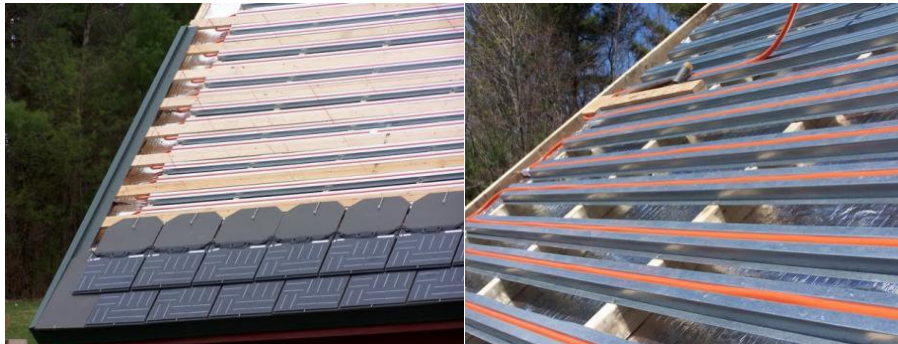
Figure 37: PV-thermal hybrid system, from Atlantis Energy Systems ( http://atlantisenergy.com ). The cells constitute a water proof roof cover. Heat is collected from the back side of the PV panels and is used for water heating.
