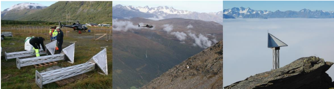
Figure 10: Overview of installation of a corner reflector in Troms County. The reflectors provide stable signal, and are covered to prevent snow accumulation.
